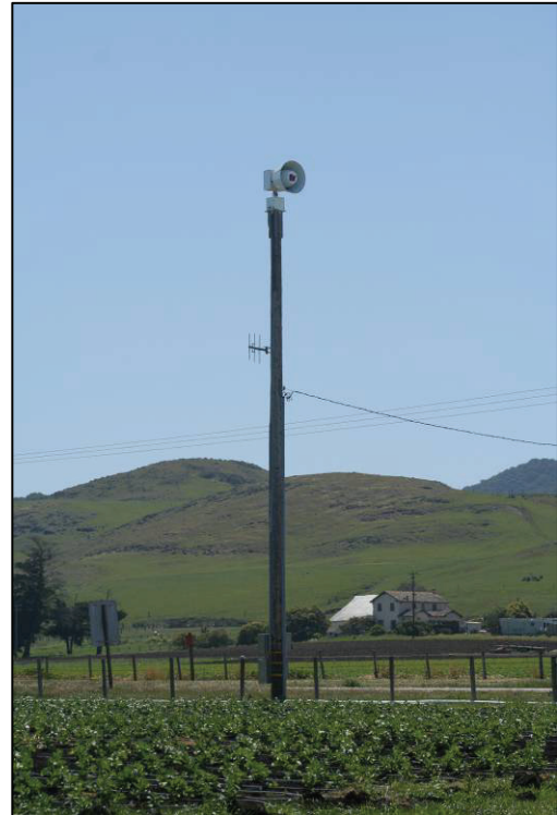
Emergency Alert Siren – Photo by Brandt Kehoe
